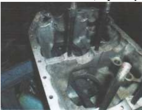
Fig 1 The crack was very hard to see With the naked eye as it was Much thinner than a human hair.
